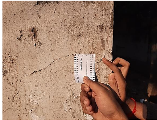
Fig. 3.10 Crack scaling during field survey.
