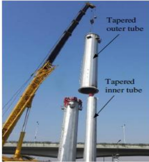
(a) High voltage pole
