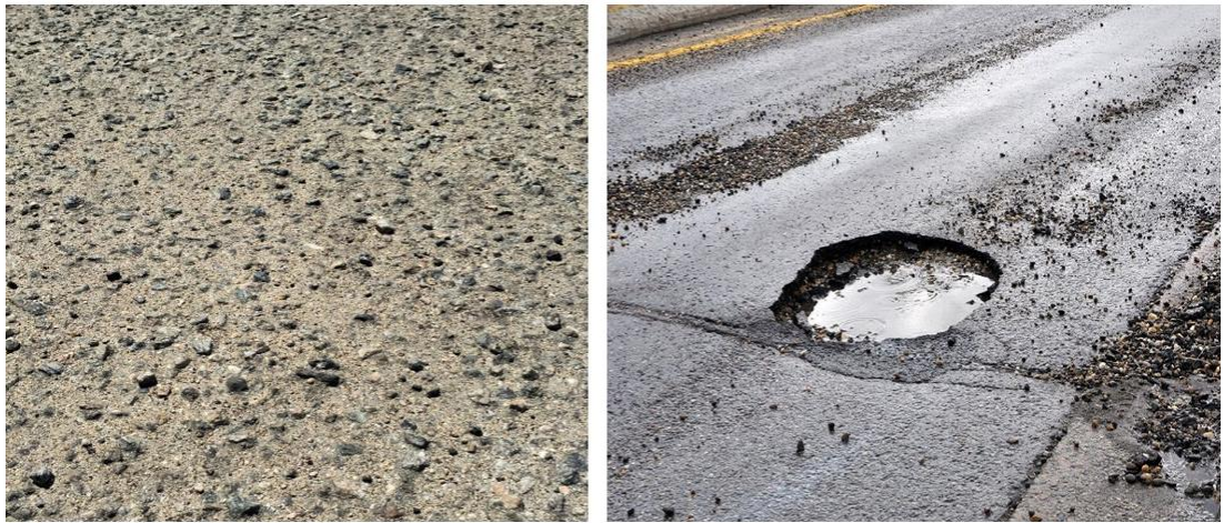
Figure 2.1: Raveling and pot hole of Pavement due to Moisture induced damage (Brown et al., 2001).
